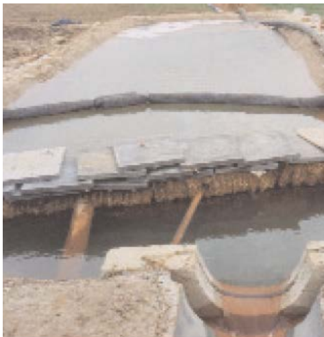
Figure 2 CIRIA 648 Settlement pond with straw bale filters and an oil boom
