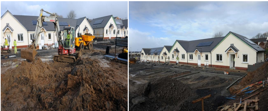
The progress being made on the bungalows in Morfa Maen, Kidwelly (7 homes)
