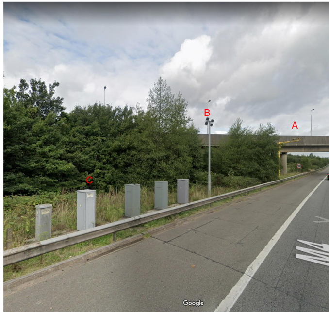
Figure 3-7. Typical ANPR camera (A), infrared lighting column (B) and cabinet (C) arrangement
