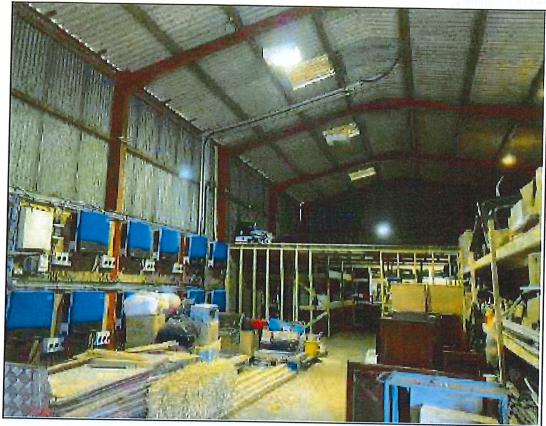
Fig. 1) Internal view of building one from Applicant's showing solar inverters and stored equipment
