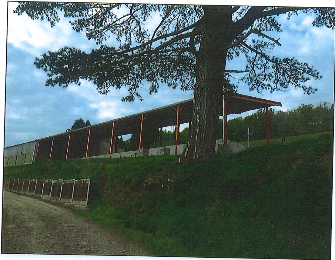
Fig. 3) Photograph taken 27th April 2022, showing prior approval works have not been implemented, although concrete block infill underway.
