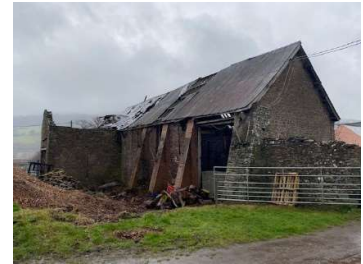
Dilapidated traditional barn
