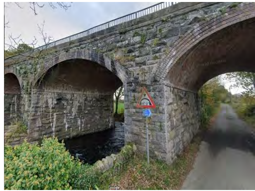
Figure 8-26 – Underside Bontnewydd Viaduct Obstruction - CD-03-04
