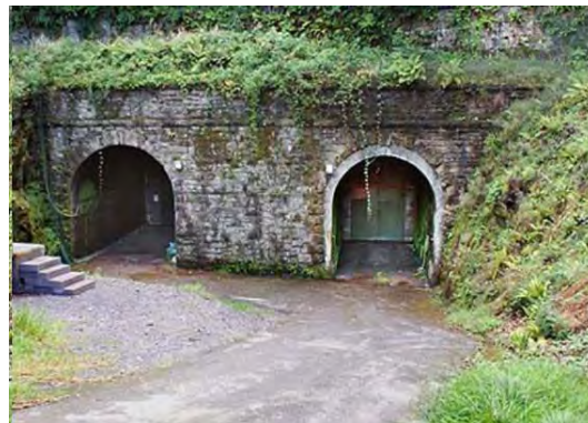
Figure 7-13 – Vaynol Tunnel Obstruction Number - BC-04-03
