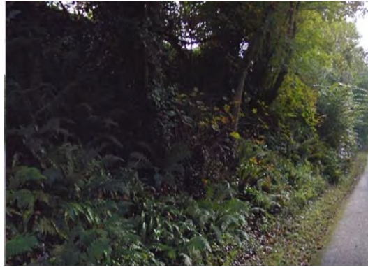
Figure 7-35 – Steep embankment Obstruction BC-07-03
