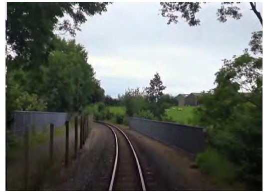
Figure 8-27 – Topside Bontnewydd Viaduct Obstruction - CD-03-04
