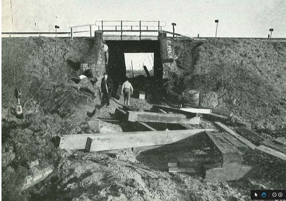
Figure 29 Sites 23 and 11 or 49. The Old Railway Bridge (Mott Hay and Anderson, 1962). The mainline (23) crossed over the mineral railways (11 and 49). This is a view at an early stage of work on construction of the A494.
