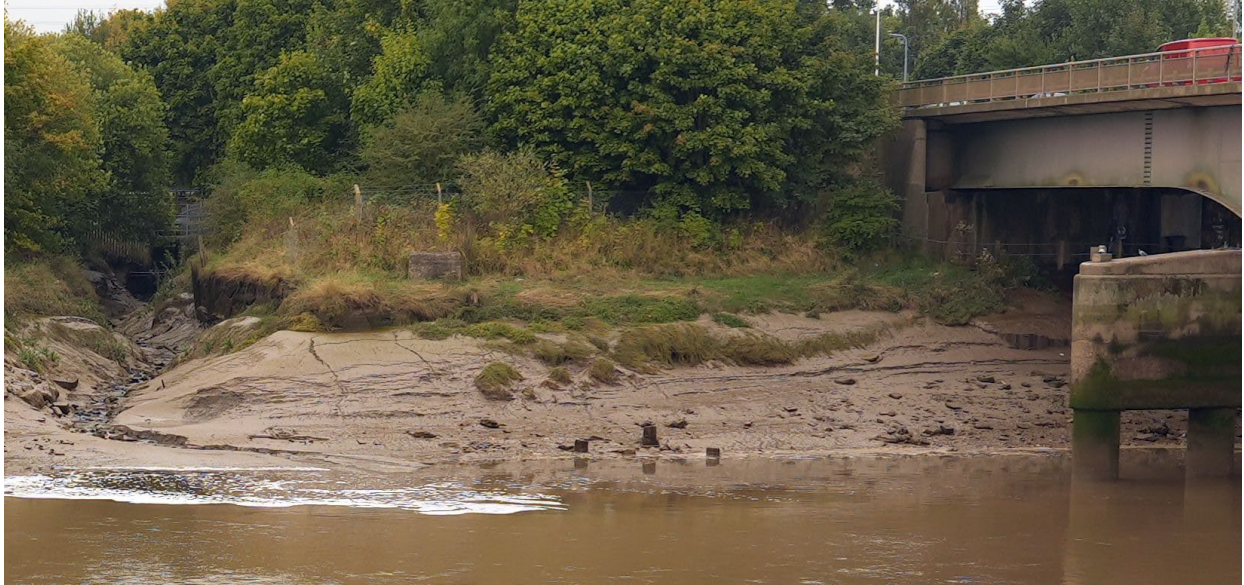
Figure 23 Concrete post bases of Site 51, Aston Quay Landing Stage III, exposed at low tide, concrete block and timber upright behind. View to the south.
