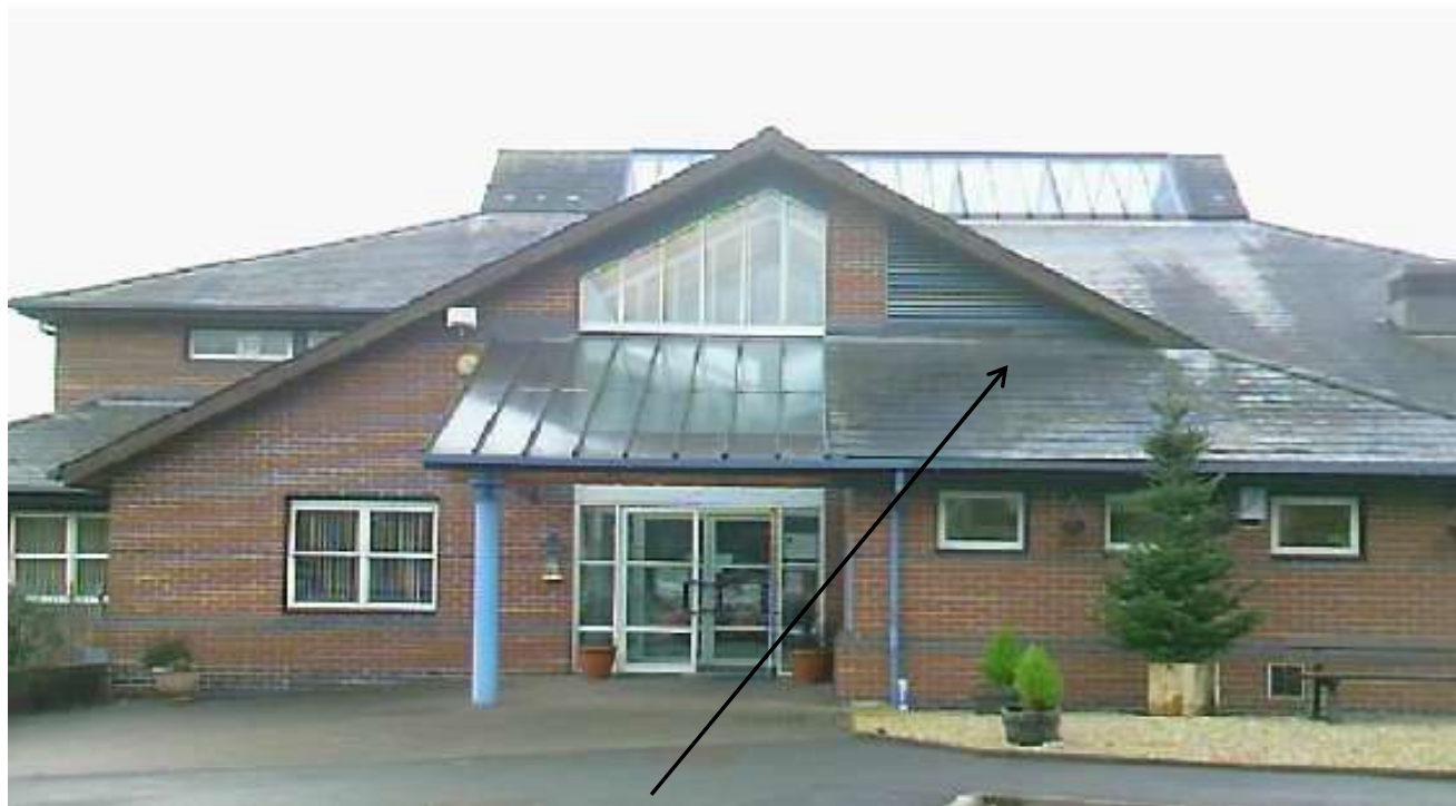
1990's to sment asbestos
