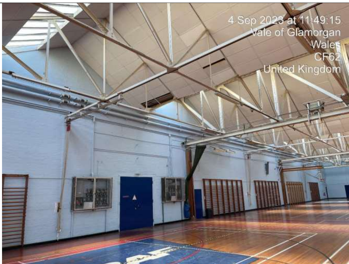
Deterioration & Missing Suspended Ceiling Tiles.
