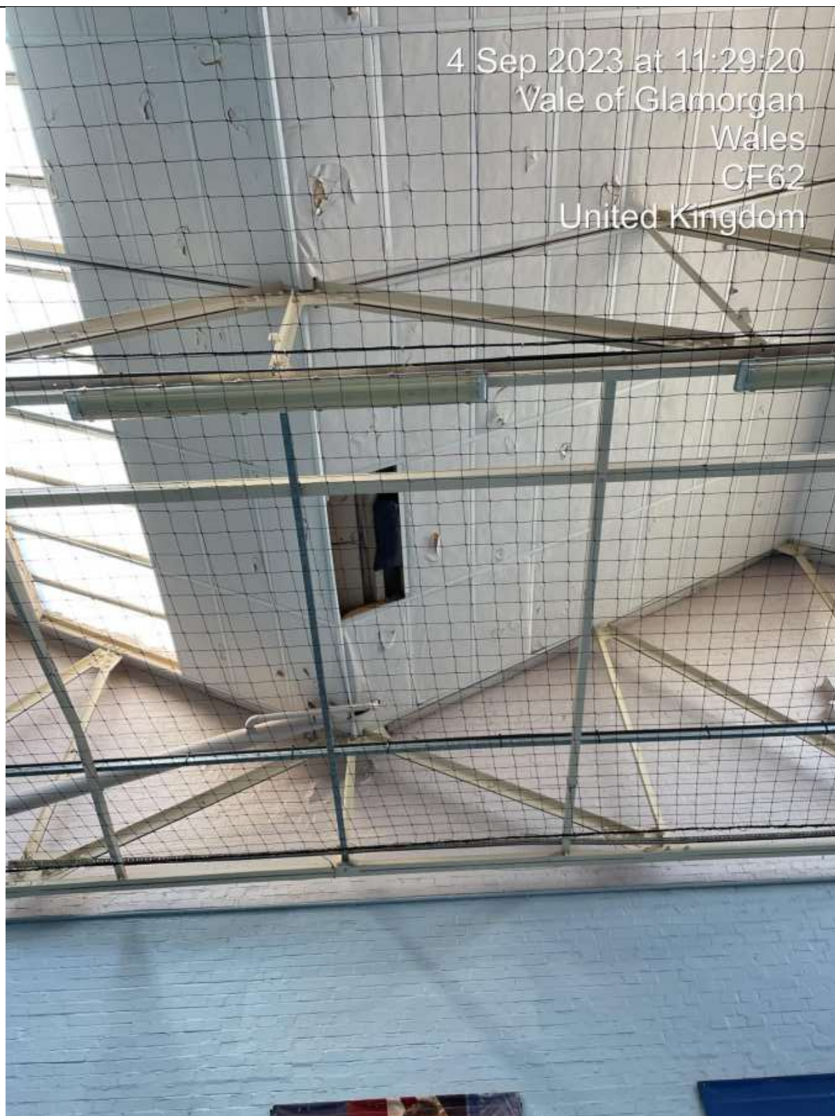
Deterioration & Missing Suspended Ceiling Tiles.
