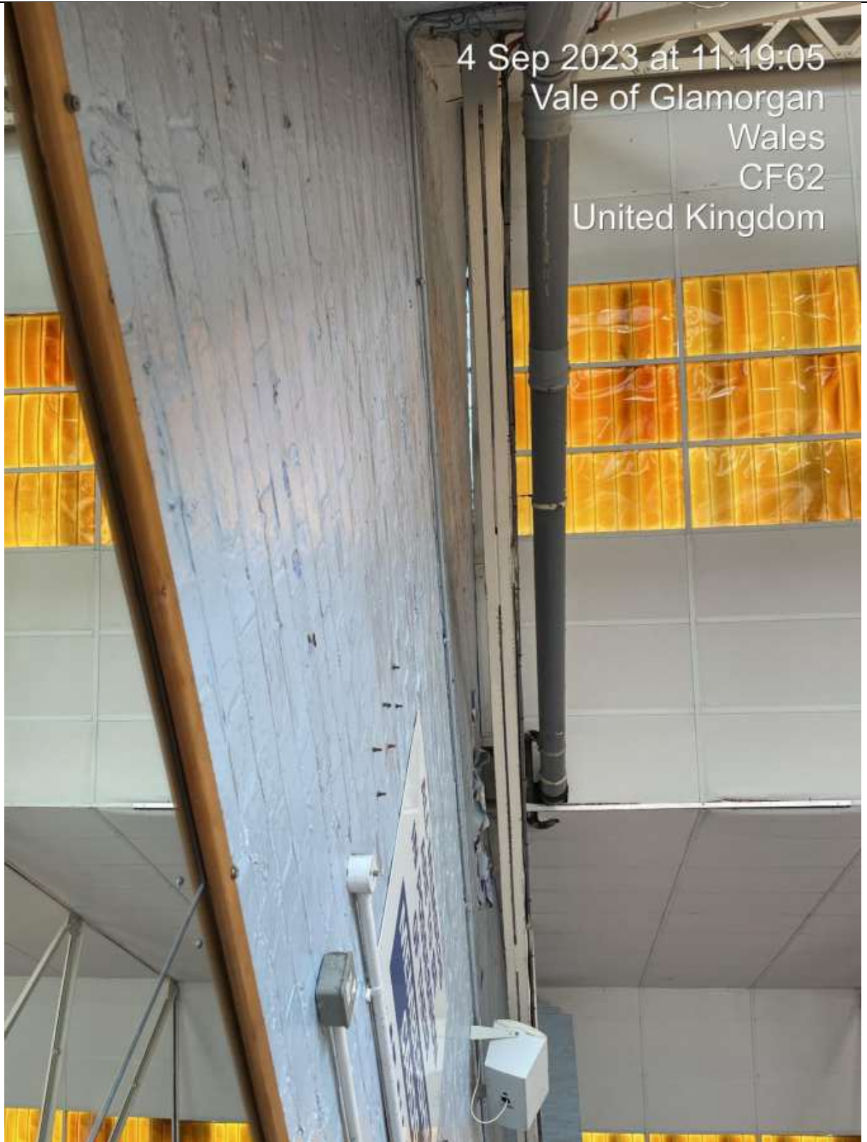
Discoloration to Roof Lights.
