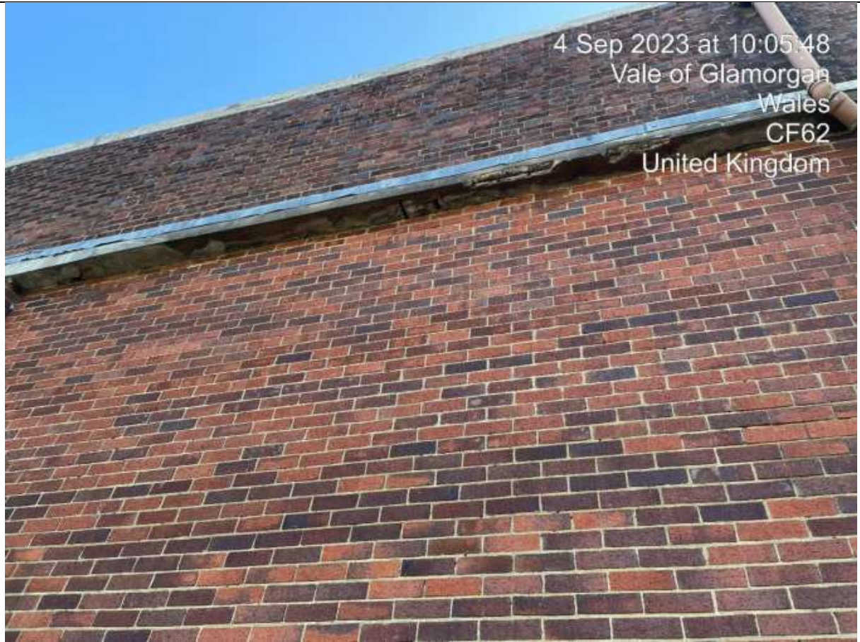
Western Elevation. Deteriation to Lintel.
