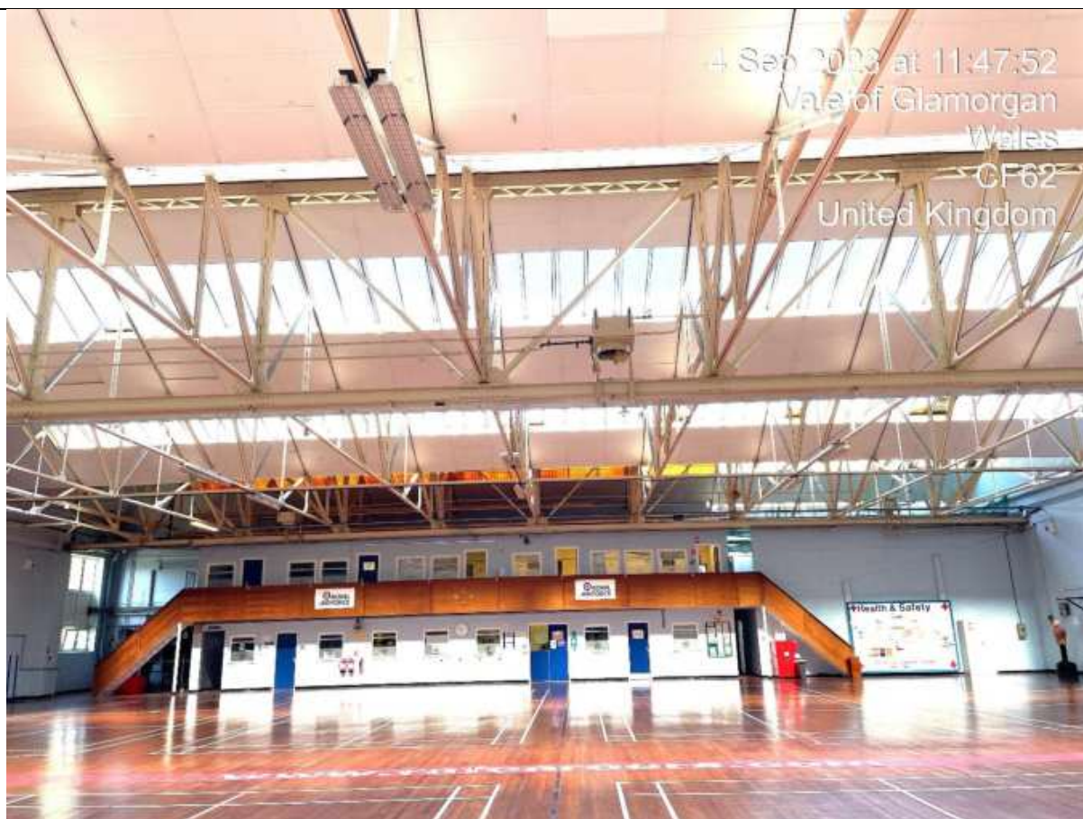
Discoloration of Roof Lights.
