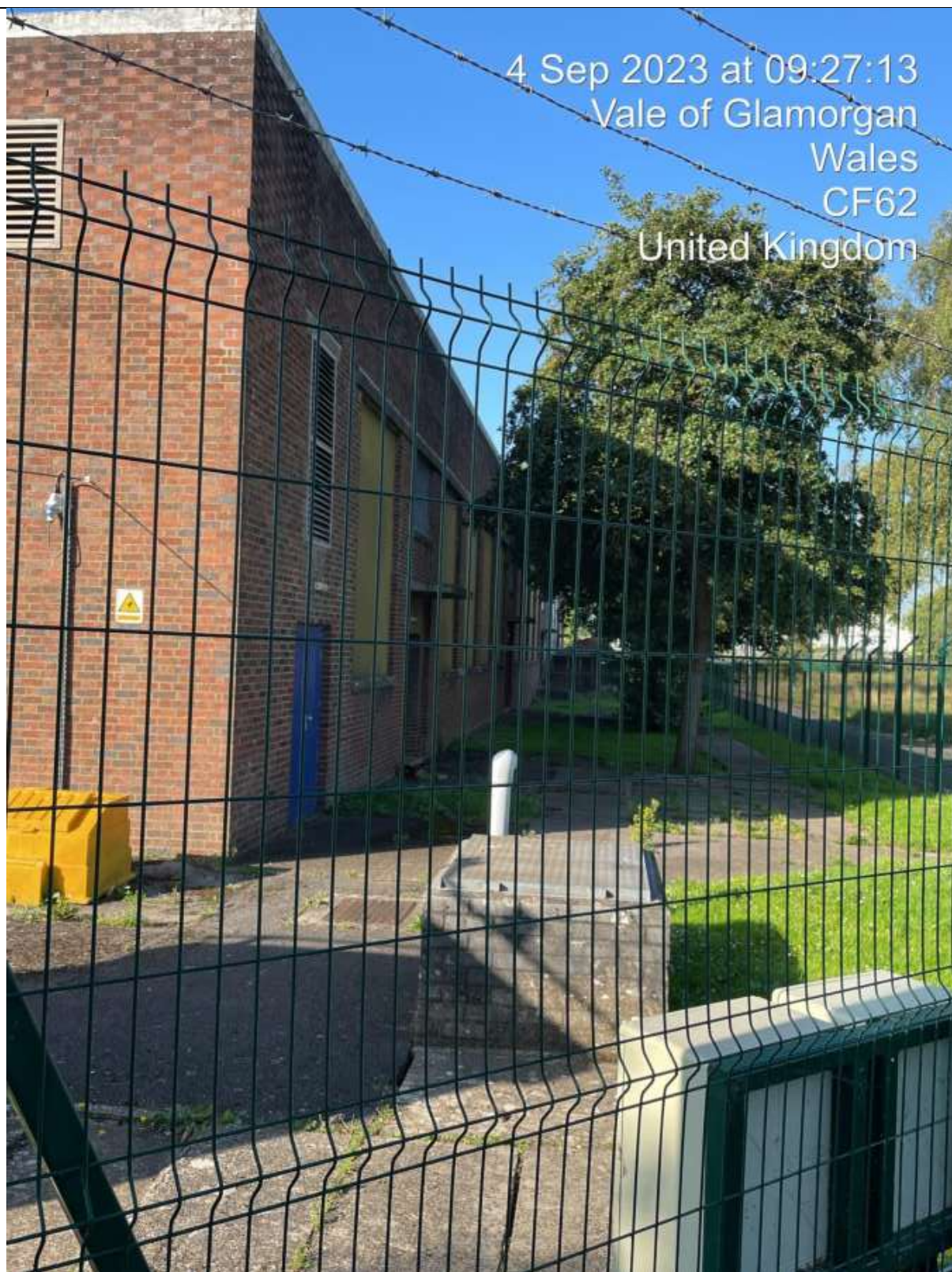
Northern Elevation. SIGNIFICANT Trip Hazards.
