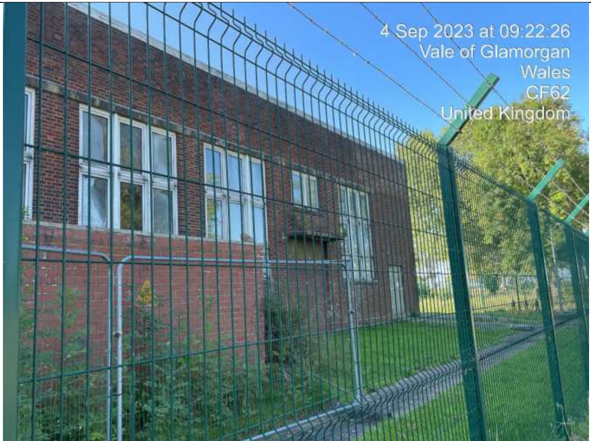
Northern Elevation. Structural Collapse.
