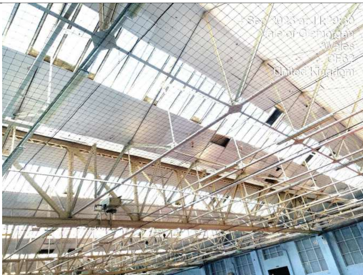
Deterioration & Missing Suspended Ceiling Tiles. Slipped Roof Lights.
