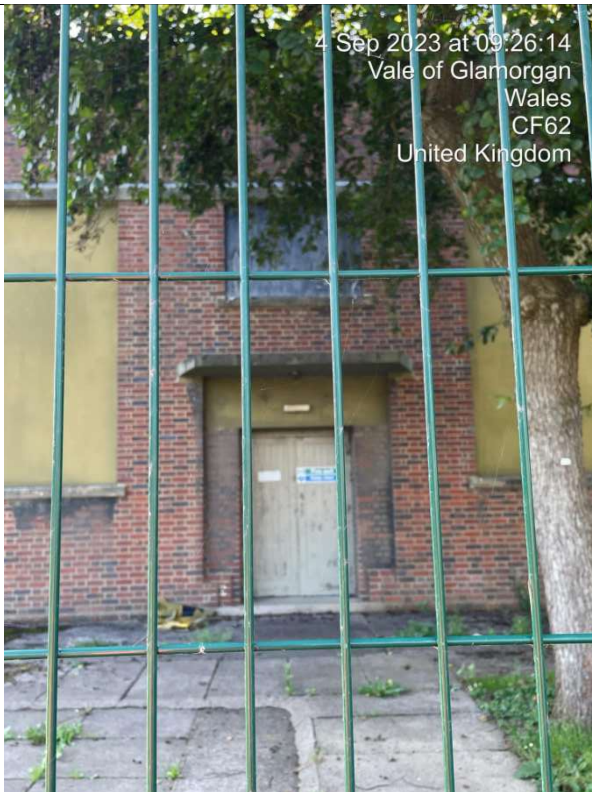
Northern Elevation. Non-Compliant Fire Exit & Trip Hazards.
