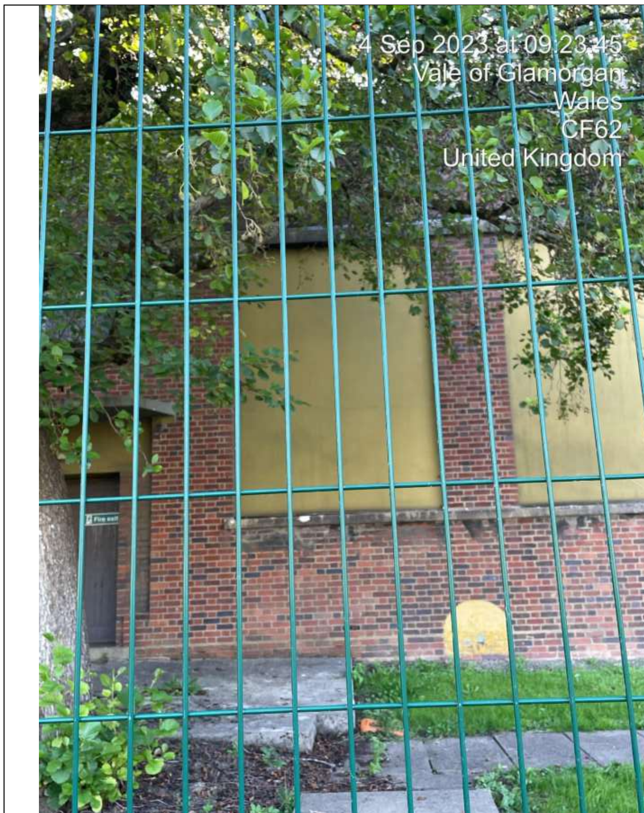
Northern Elevation. Blanked Off Fenestration and Trip Hazards to Path.
