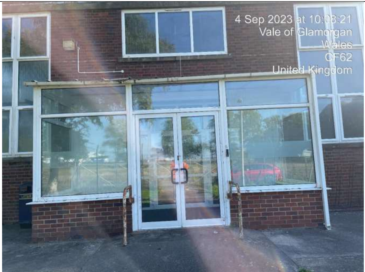
Western Elevation. Later Entrance Porch that is Non-Compliant.
