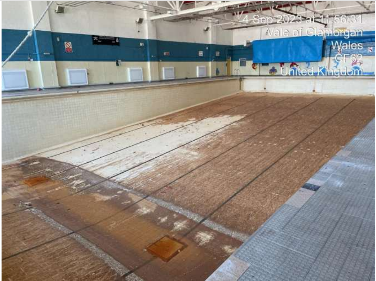
Empty Swimming Pool with Residual Contamination.
