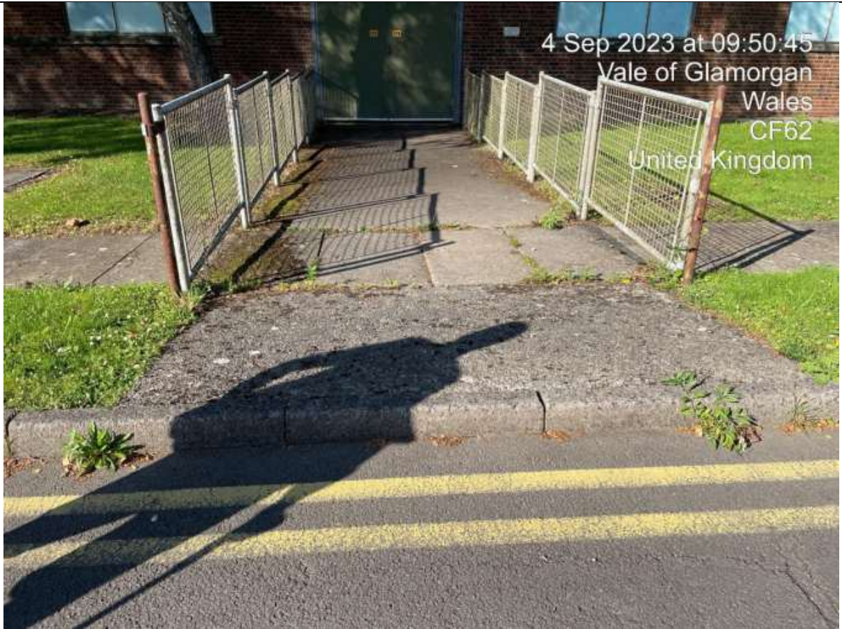
Eastern Elevation. Non-Compliant Access & Egress.
