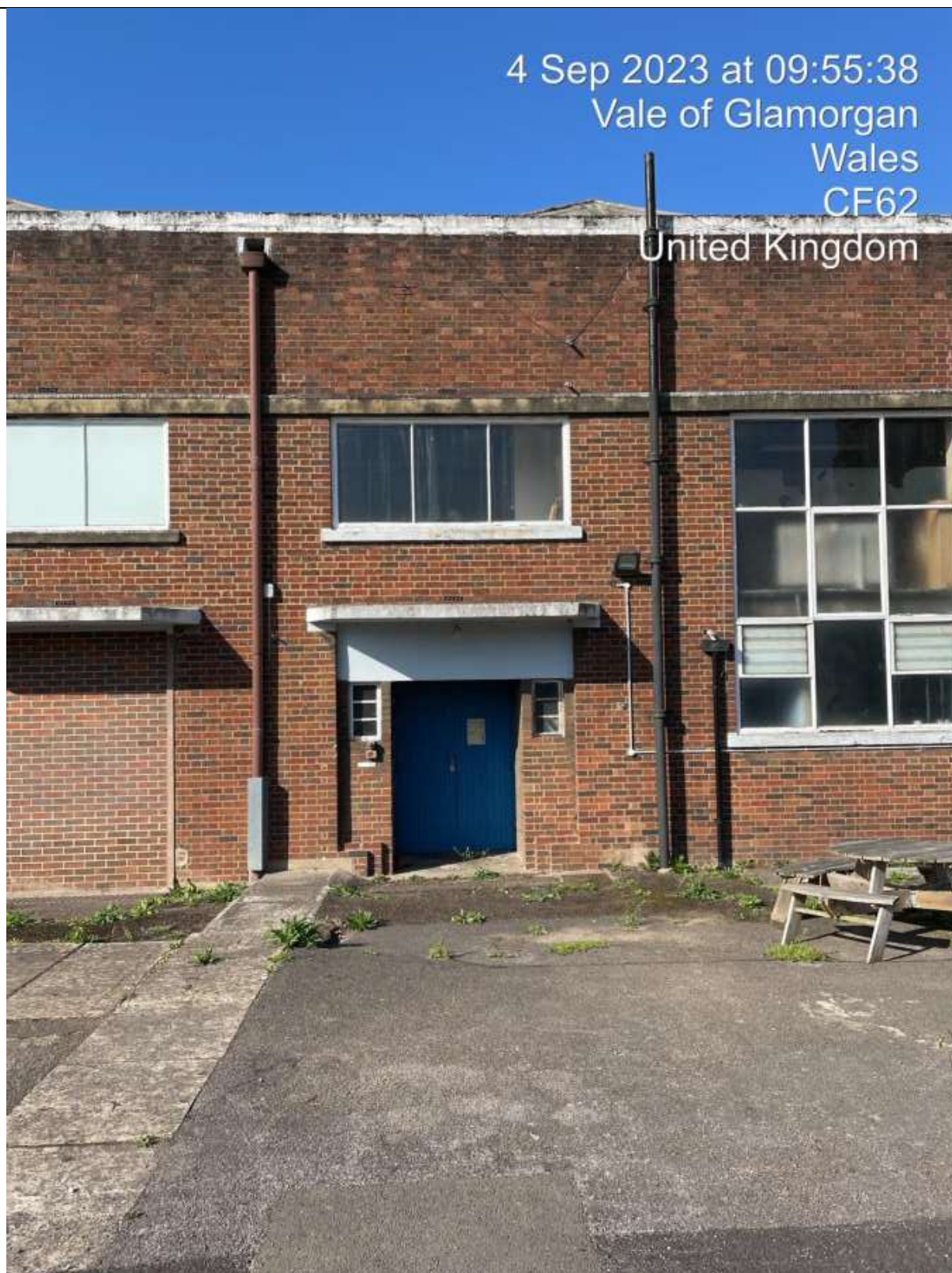
Eastern Elevation. Deterioration to Doors.
