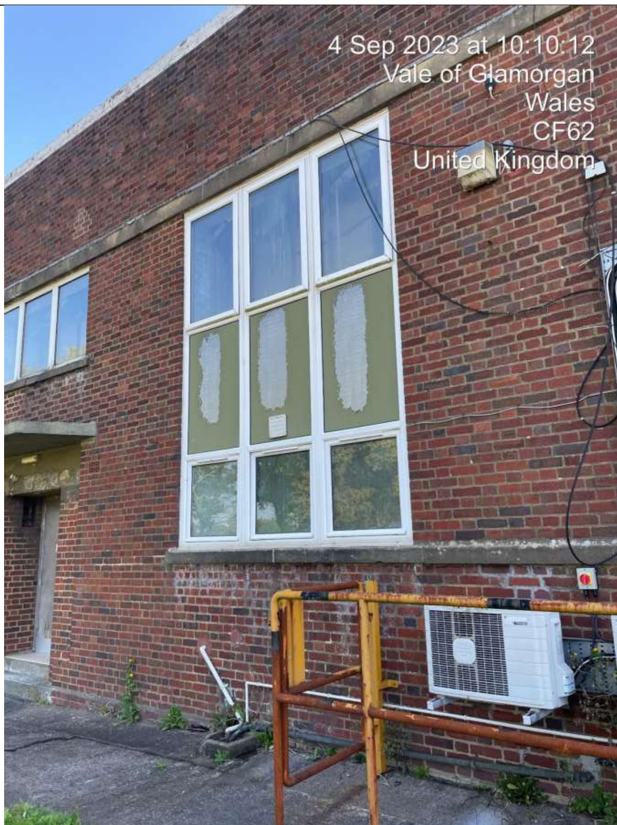
Western Elevation. Replacement Fenestration that is Deteriorating.
