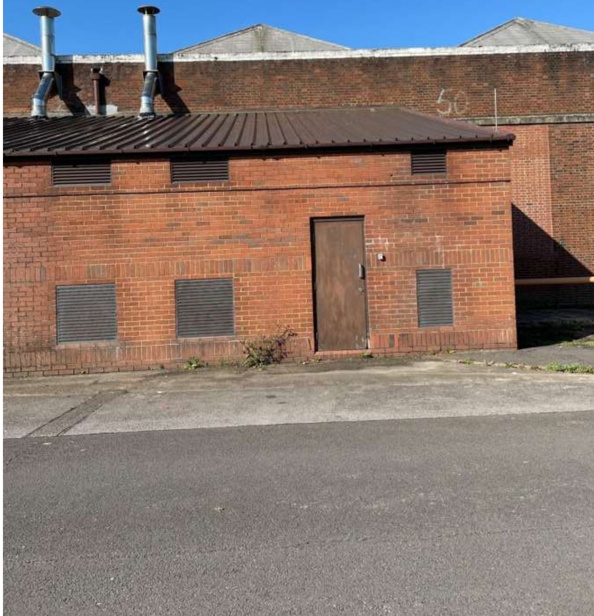
Eastern Elevation. Non-Original Plant Room Addition with Deterioration to Door.
