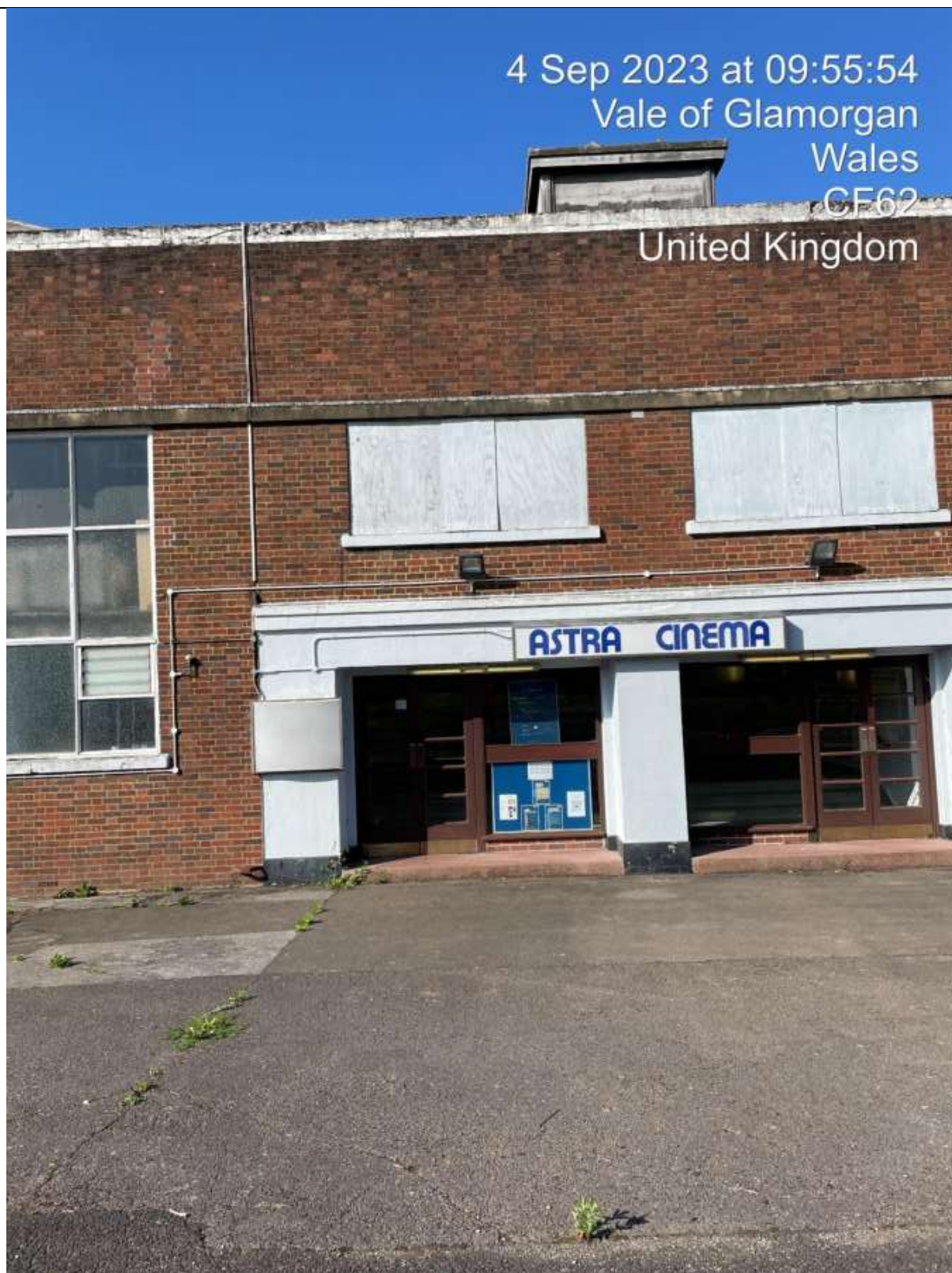
Eastern Elevation. Non-Compliant Access & Egress Points.
