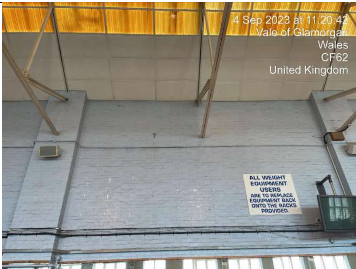
Discoloration to Roof Lights.
