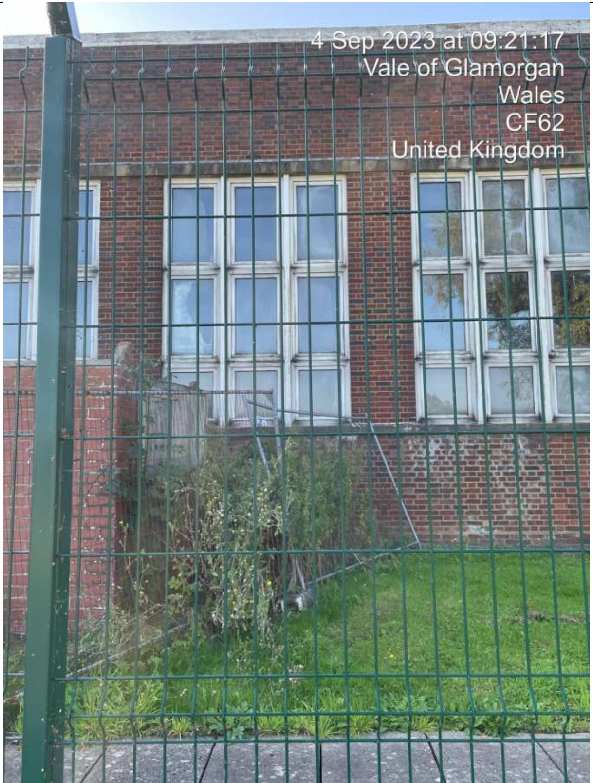
Northern Elevation. Structural Collapse.
