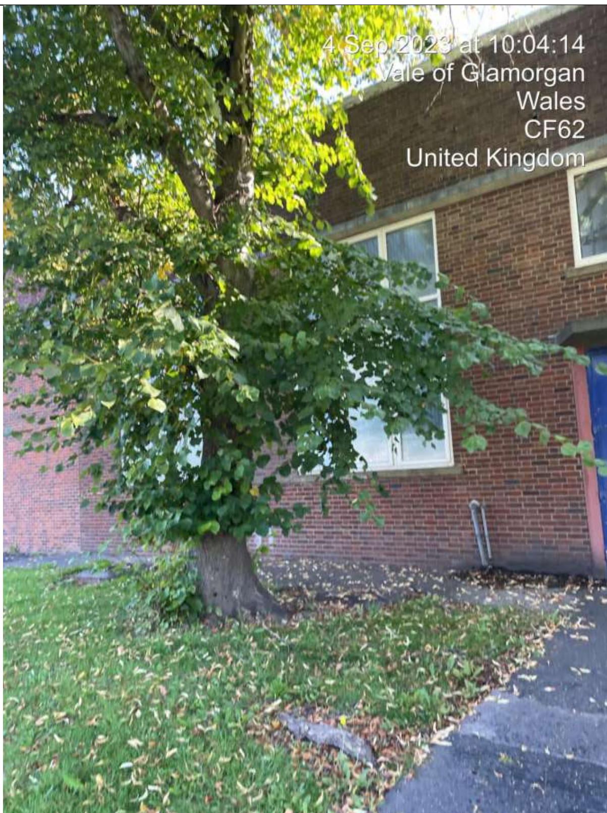
Western Elevation. Proximity of Trees to Building cause suspect of Damage to Foundations.
