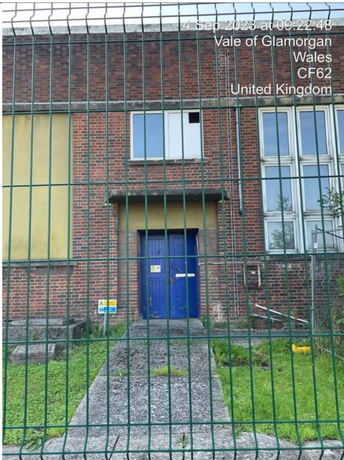
Northern Elevation. Deterioration of Plant Room Doors.
