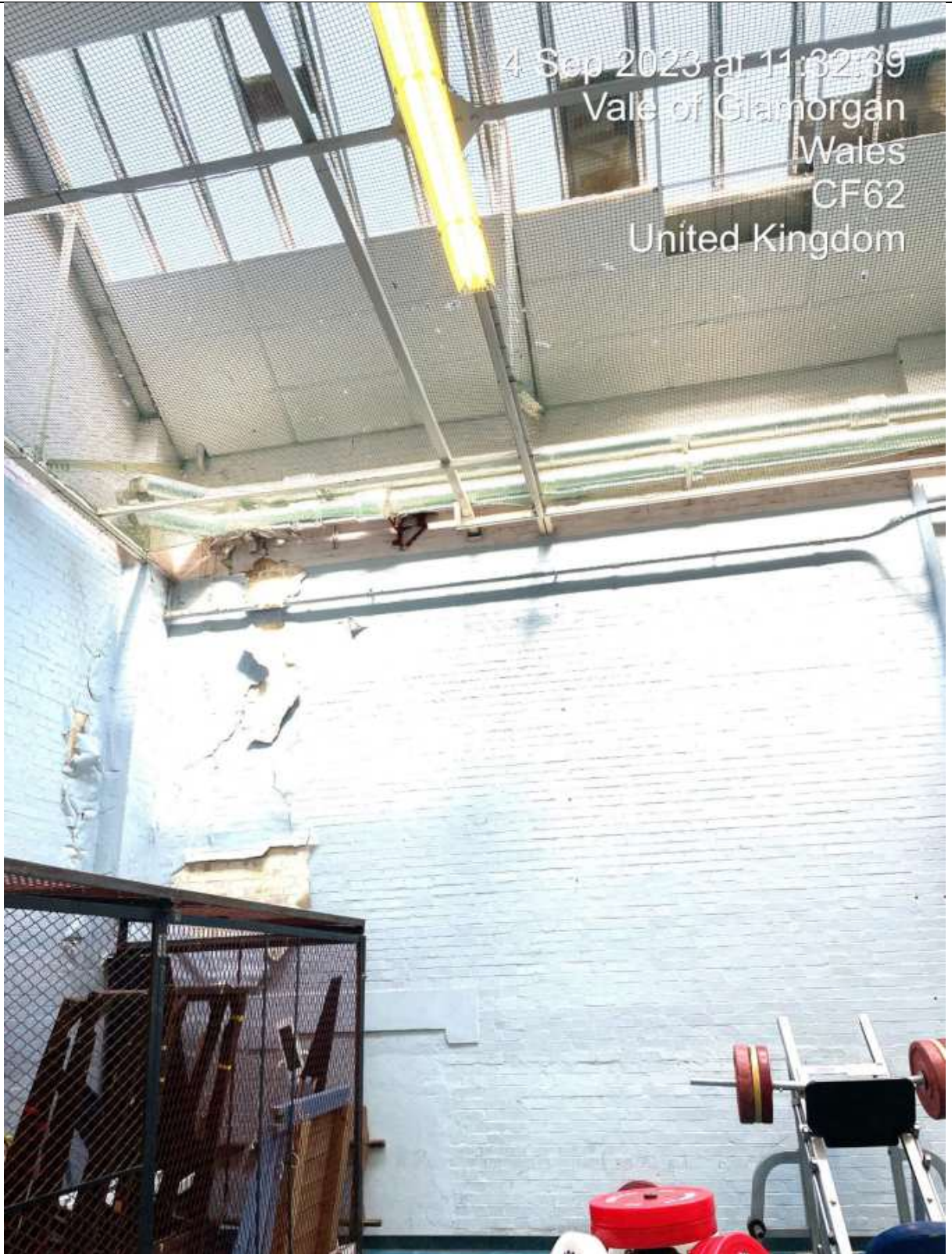
SIGNIFICANT Penetrating Damp.
