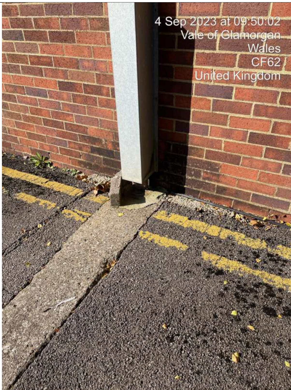
Eastern Elevation. Downpipe from Hidden Gutter NOT PENETRATING TO DRAINAGE.
