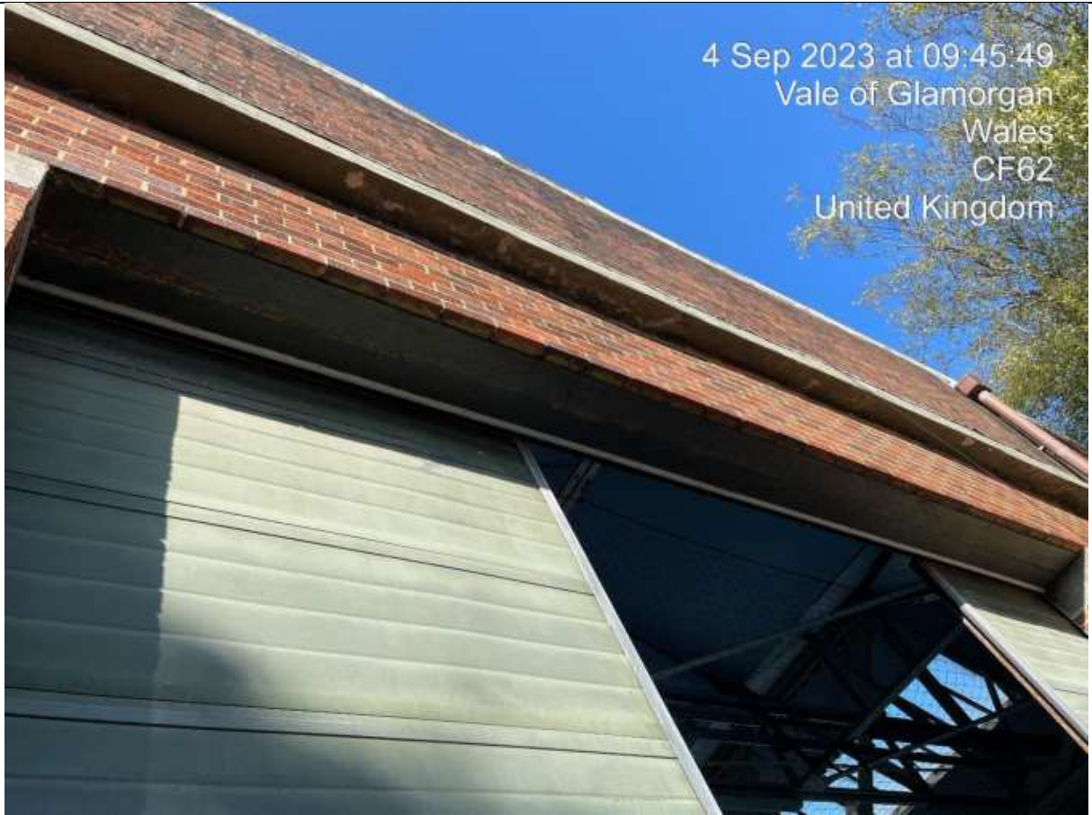
Eastern Elevation. Corrosion to Replacement Steel Lintel.
