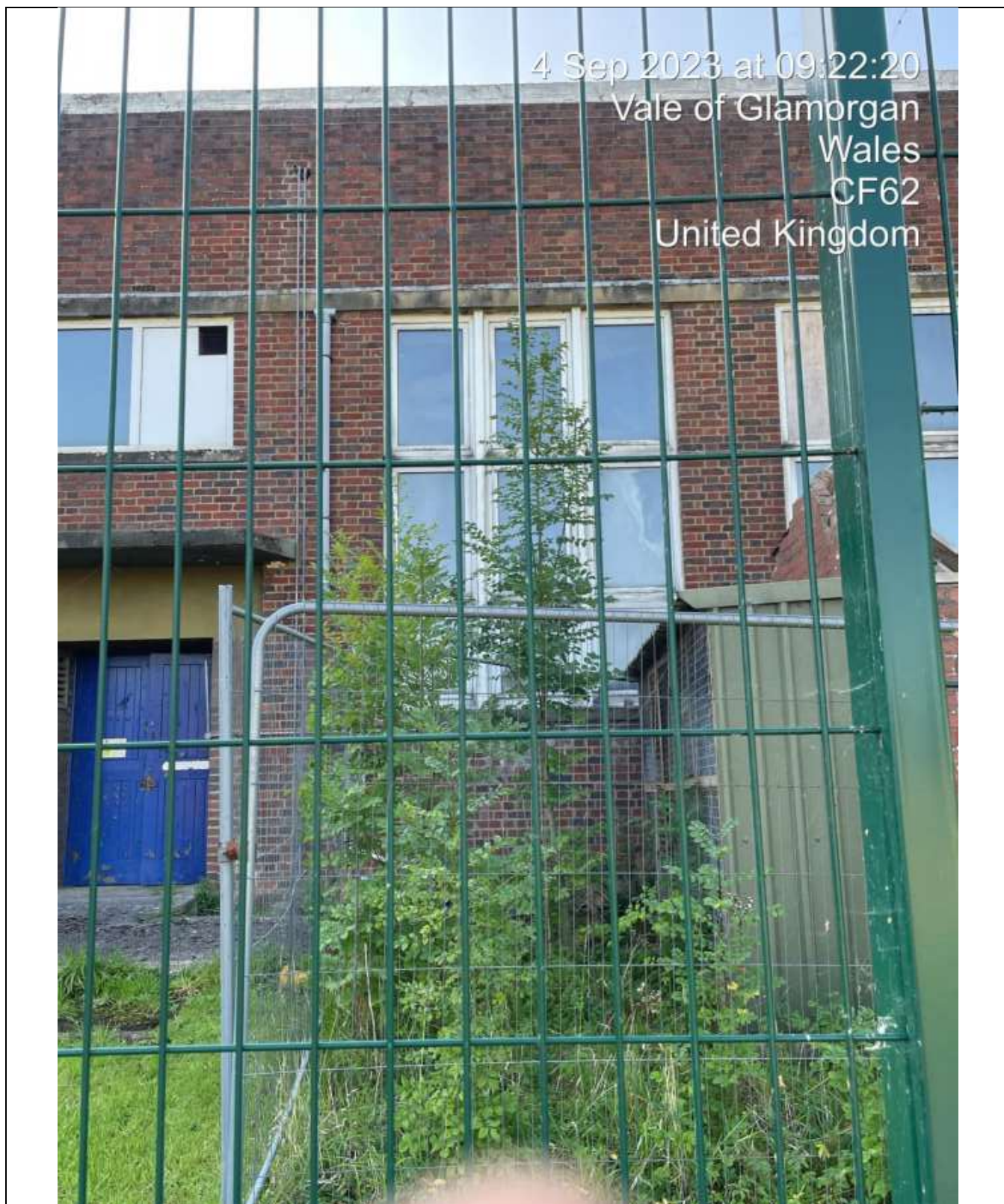
Northern Elevation. Structural Collapse.
