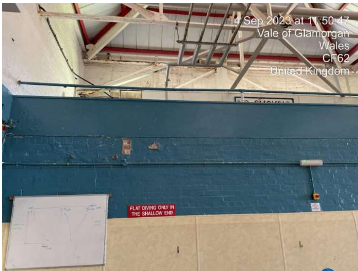
Corrosion to Steel Roof Frame & Penetrating Damp.
