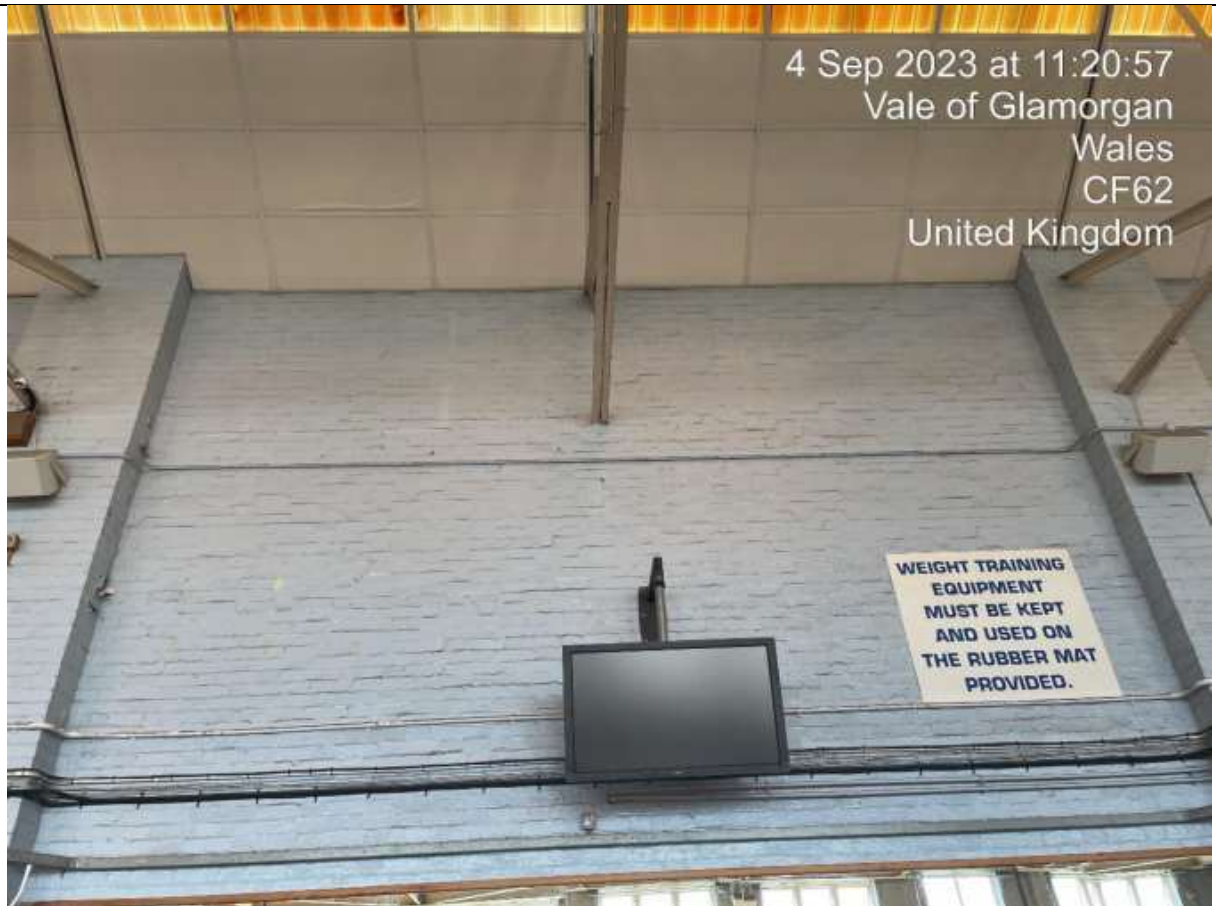
Penetrating Damp & Unprotected Cable Installations.
