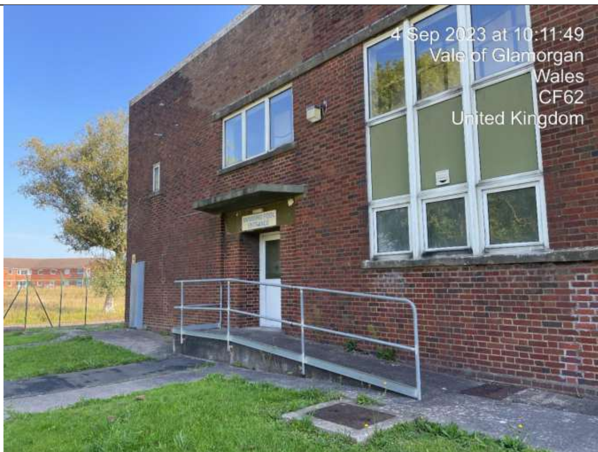
Western Elevation. Swimming Pool Entrance. Note Non-Compliant.
