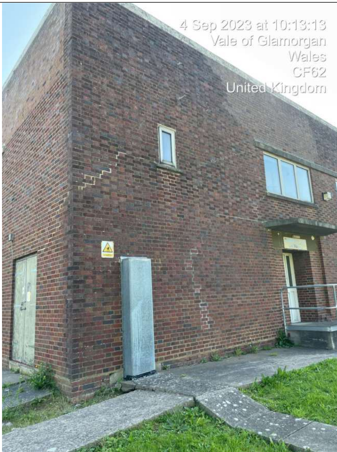
Western Elevation. Significant Brickwork Replacement Demonstrating Structural Movement & Structural Rotation.
