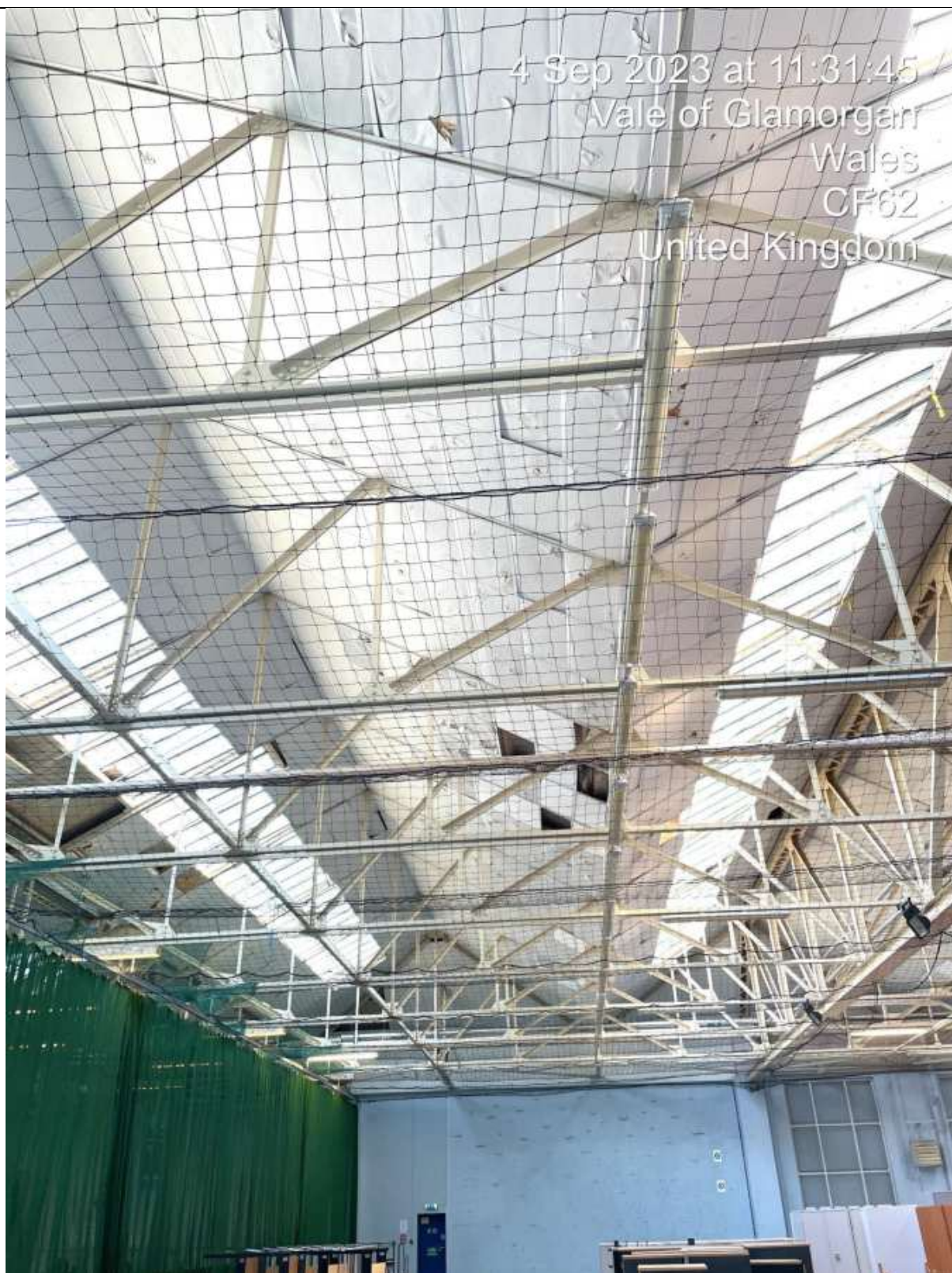
Deterioration & Missing Suspended Ceiling Tiles.
