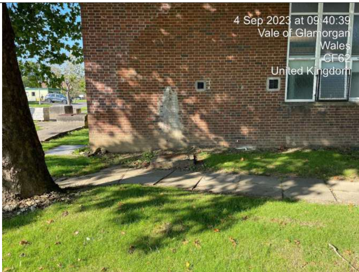
Eastern Elevation. SIGNIFICANT Trip Hazards to Footpath.
