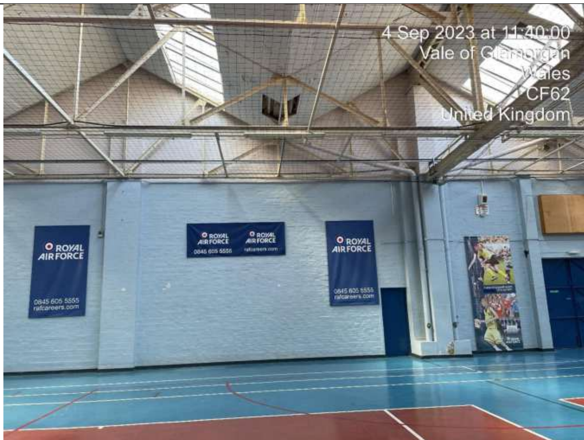
Deterioration & Missing Suspended Ceiling Tiles.
