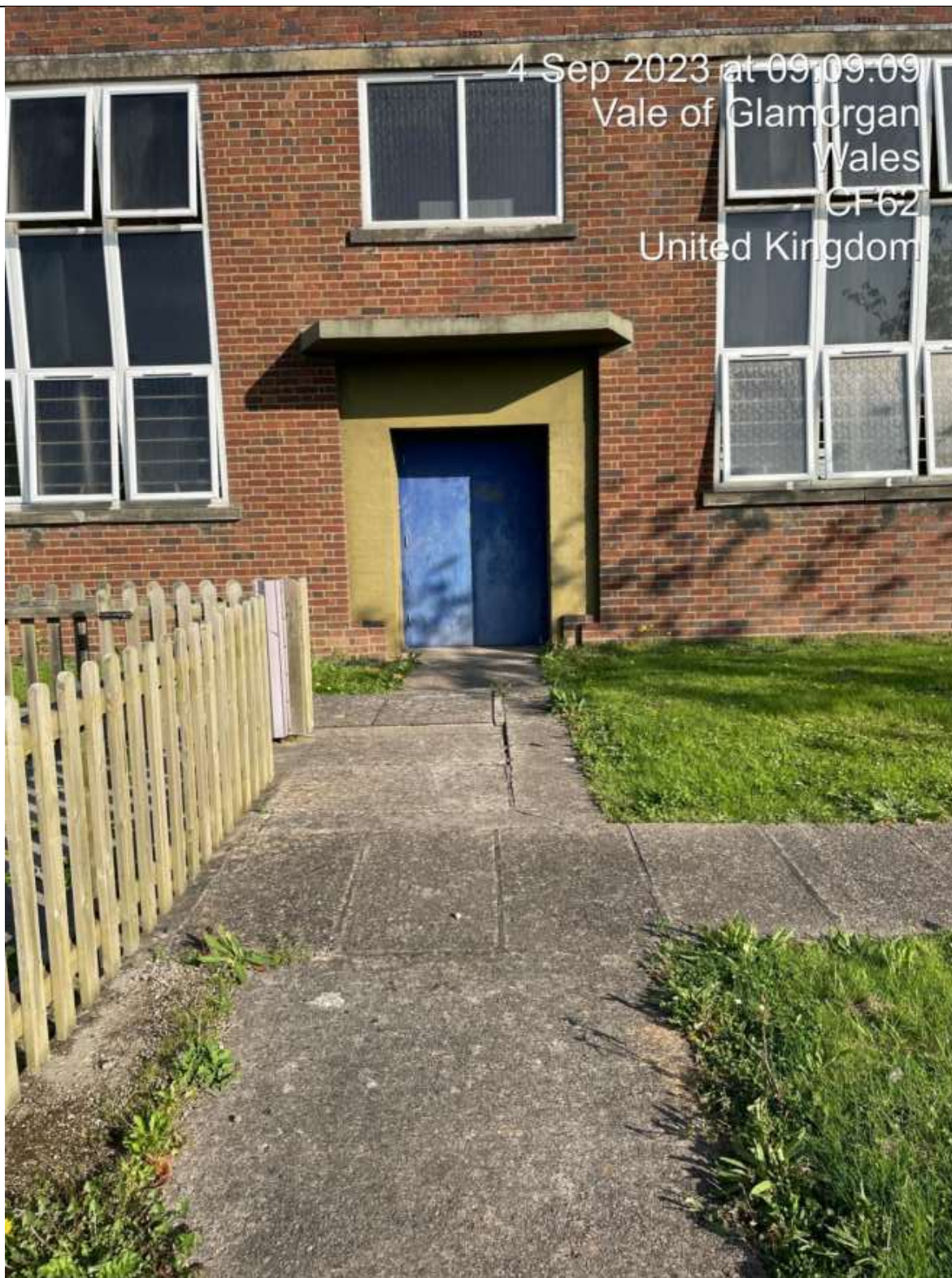
Southern Elevation. Non-Compliant Entrance with Trip Hazards.
